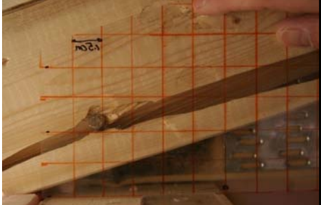
Example of a toe-nail roof to wall connection in the house where the nail has split the wood and offers very little hold down force.
