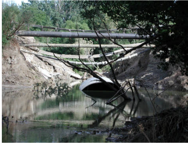
Figure 2: Toronto's Finch Avenue after the August 19, 2005 Storm
